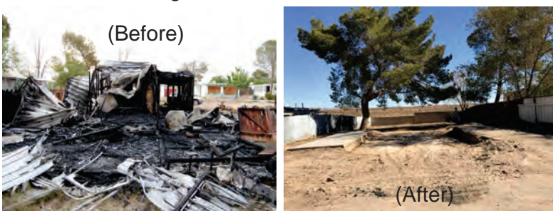
Dangerous Structure Demolished
